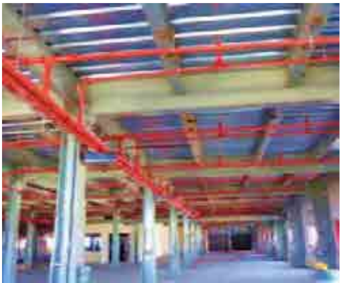
Automatic Foam Sprinkles System installed with QBD & IR3 detection
